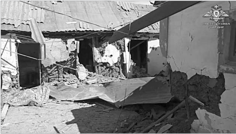
In the photo the consequences of the shelling of the Petrovsky District of Donetsk, 1 Velyaminov Street, which resulted in the death of a man of 1978 year of birth
